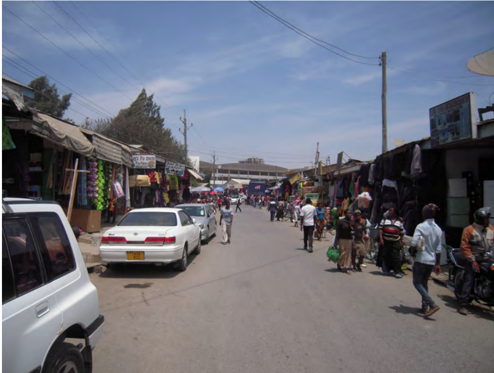
Figure 10. Mwanjelwa Market Street and the building site of the shopping mall in the background (Mbeya)
