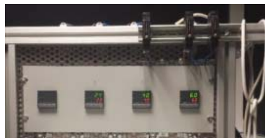
Fig. 4. Temperature controllers and meters (in hours)
