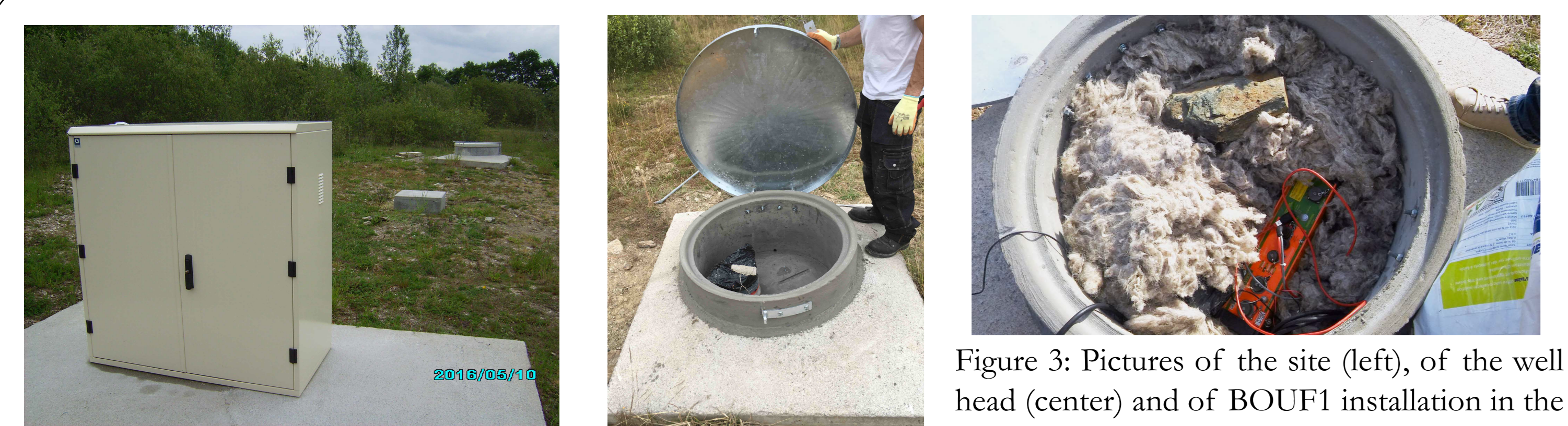
Figure 2: Borehole is instrumented with a T120PH (BOUF) surrounded by sand (right). A T120PA (BOUF1) was installed at the surface in the concrete pipe that covers the well (left).
