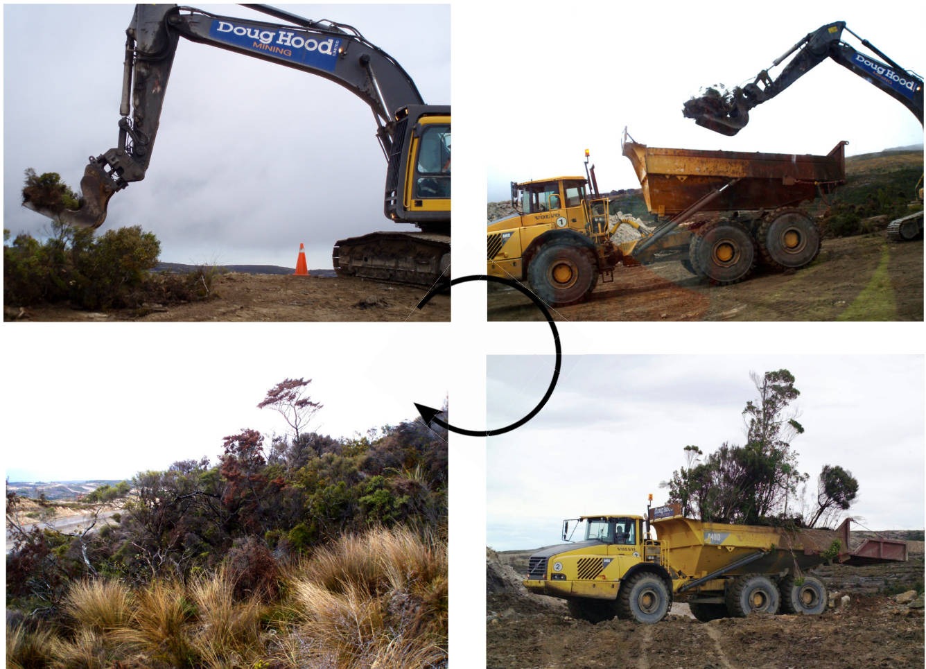
Figure 1. Vegetation direct transfer of native alpine forest at the Stockton opencast coal mine (New Zealand). Clockwise: pieces of land comprising vegetation, roots and soil are cut; soil and vegetation sods are loaded on a truck and transported to the receptor site; the landscape jigsaw is then reconstituted with minimum gaps between the sods to recreate a continuous habitat. Credits: Stéphane Boyer and Solid Energy New Zealand Ltd.
