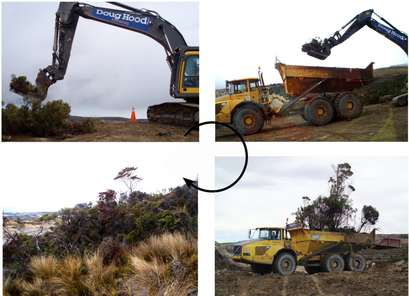
Figure 1. Vegetation direct transfer of native alpine forest at the Stockton opencast coal mine (New Zealand). Clockwise: pieces of land comprising vegetation, roots and soil are cut; soil and vegetation sods are loaded on a truck and transported to the receptor site; the landscape jigsaw is then reconstituted with minimum gaps between the sods to recreate a continuous habitat. Credits: Stéphane Boyer and Solid Energy New Zealand Ltd.
