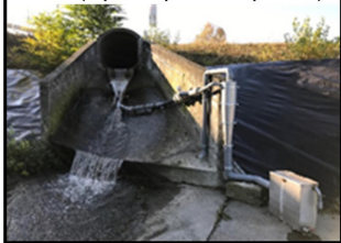
Inlet (hydrocyclone system)
