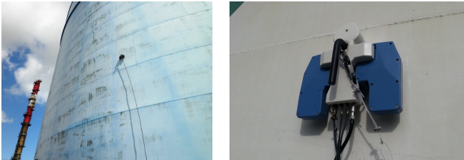
Fig. 1. Typical inspection conditions for magnetic crawlers operating on a structure assembled out of welded steel plates [Source: RoboPlanet]
