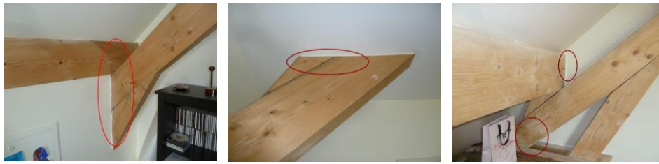
Figure 6: leakages at the junctions between the wood frame and the ceiling or the walls
