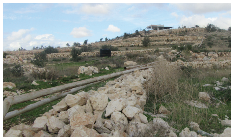
Pipes laid at the farmer’s expense to irrigate these terraces high in the mountain
