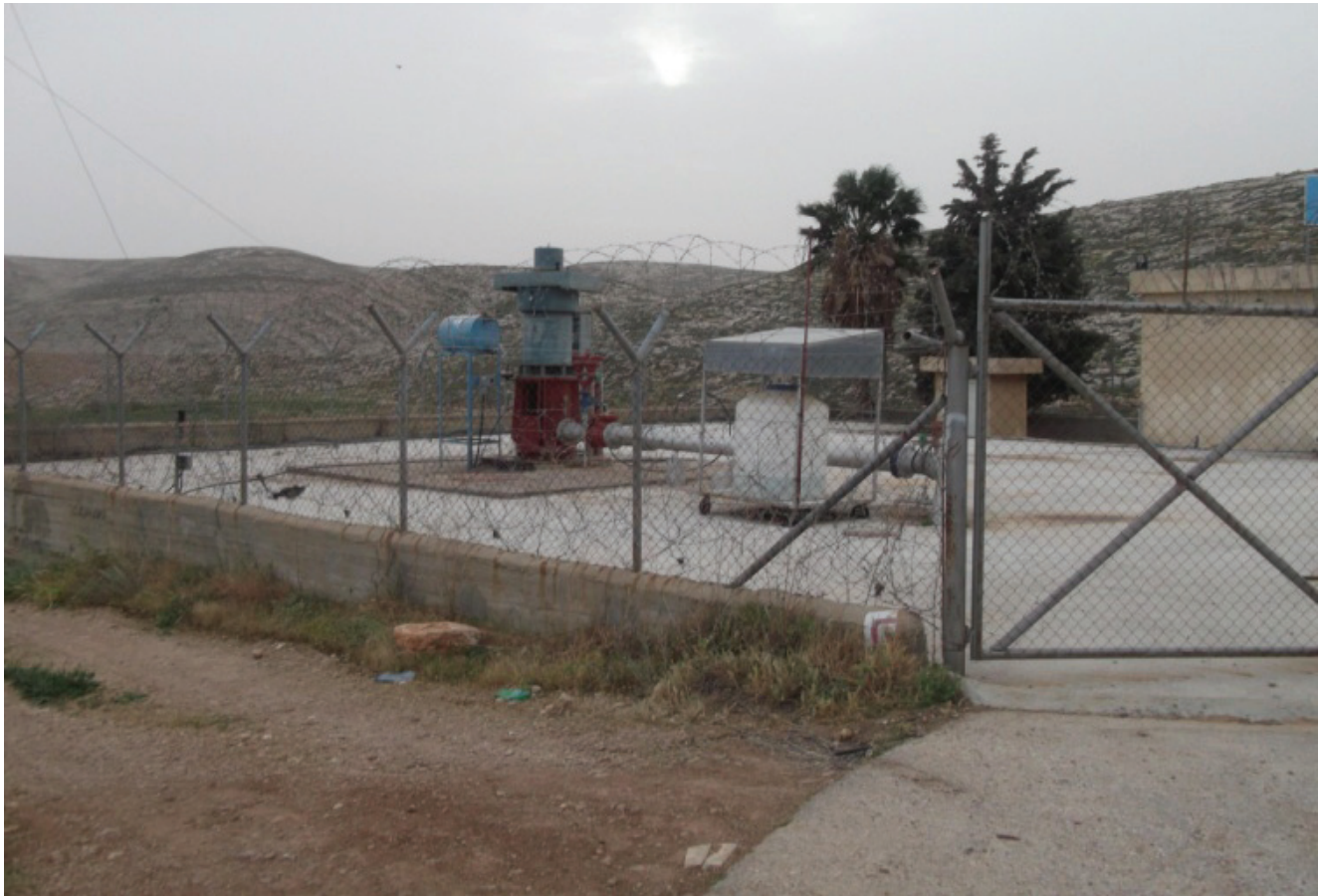
Well suspected of interfering with Al-Auja Spring (2013)
