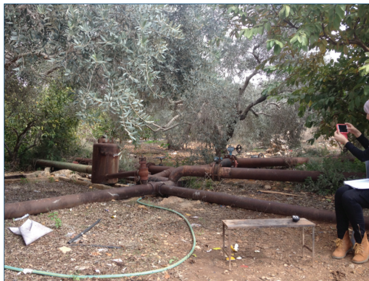
Pipes leading to fields from an agricultural well
