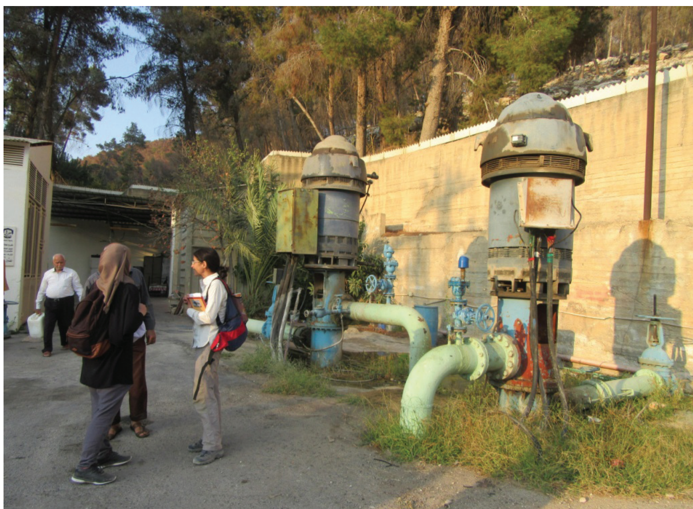
Boosters at Al-Badan pumping station operated by the Municipality of Nablus
