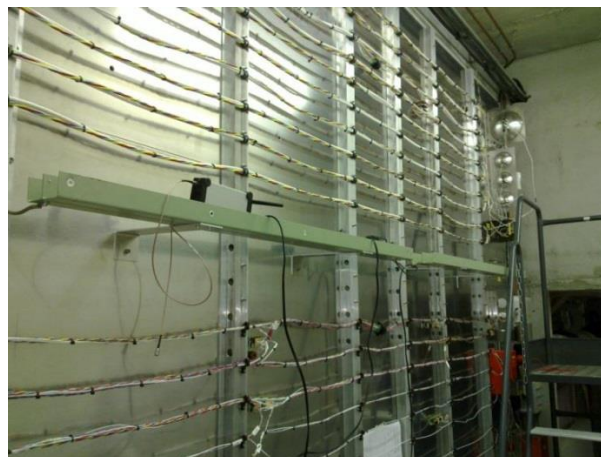
Figure 5 : ON-LINE bench, equipped with real loads (lights, etc), powered by a real aircraft generator
