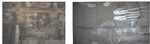
Figure 1: Examples of images of the sidewall of a masonry tunnel (left) and the vault of a concrete tunnel (right)
