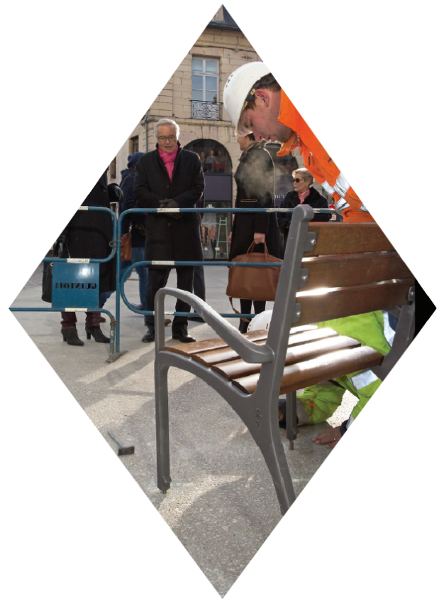
Figure 7. Installation of a bench under the supervision of a Mayor. The promotional document here refers to “A participatory democracy challenge”. Source : Lefebvre and Chapon (2014, p. 38).
