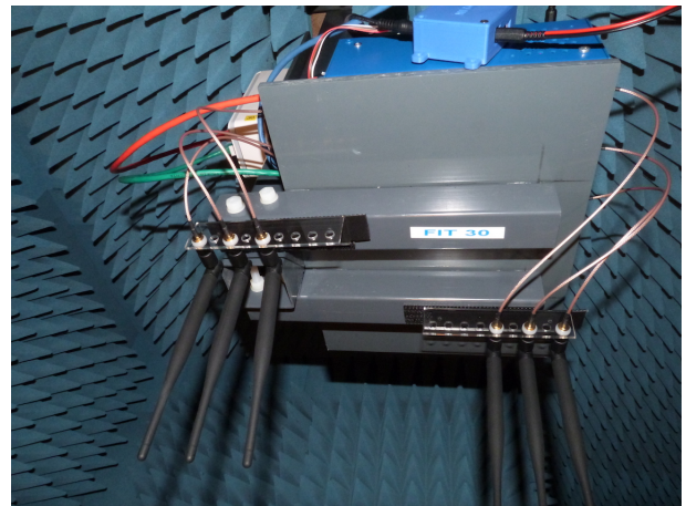
Figure 3: Wi-Fi dual-band antennas for a node
