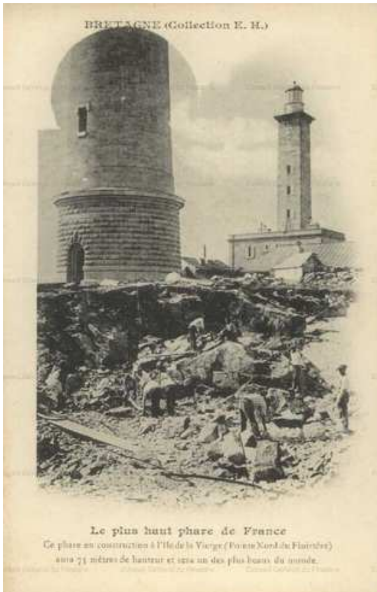
Figure 6 - Extraction of granite at the foot of the Ile Vierge lighthouse [A8]
