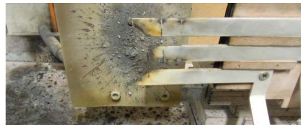
Fig. 1 Example of busbars after arcing [1]
