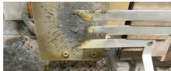
Fig. 1 Example of busbars after arcing [1]
