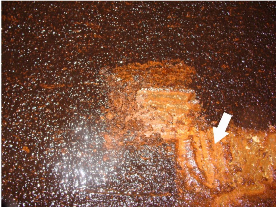
Fig. 2. Biofilm on the concrete HR Tunnel. The white arrow indicates biofilm removal after sampling.
