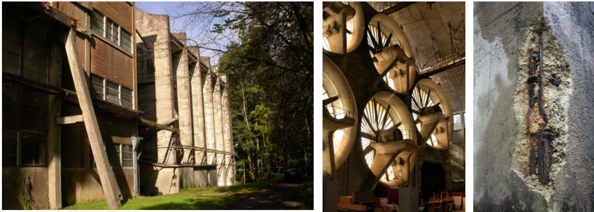
Figures 1, 2 and 3 : The air purifier (on the left) is an extension of the Meudon wind tunnel (in the center). It is locally very decayed, with large spalling areas (on the right) often linked to honeycombing.
