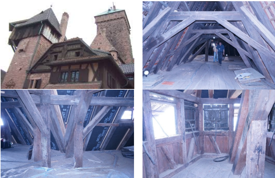
Figure 3. Castle of Haut-Kœnigsbourg (top left) and details of its truss structure (top right and bottom).
