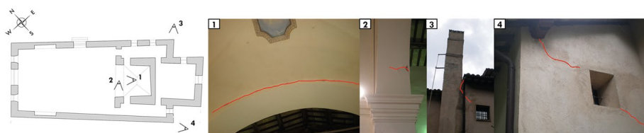
Fig. 11 Damage survey in Madonna of Valcora Sanctuary in Fiuminata after the Central Italy Earthquakes of 2016
