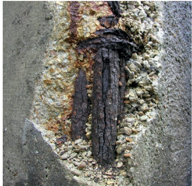
Figure 2: Concrete spalling observed on ONERA site
