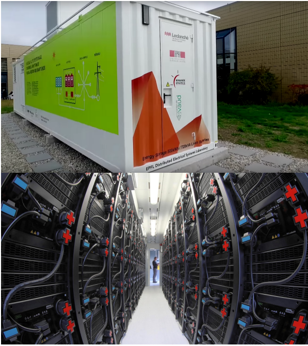
Fig. 8. An outside (top picture) and inside view (bottom picture) of the 720 kVA/500 kWh Lithium Titanate-based BESS used in this experimental work. The system, developed by Leclanché, includes a four-quadrant fully controllable DC/AC converter and a 0.3/20 kV step-up transformer. It is hosted in a temperature controlled container (picture of Alain Herzog, EPFL).
