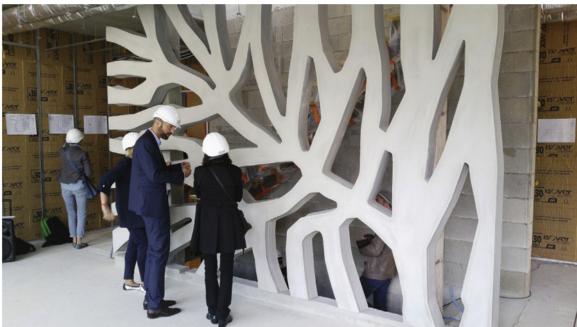
Figure 3.16 Interior wall made of the 3D-printed concrete formwork filled with cast concrete after finishing.
