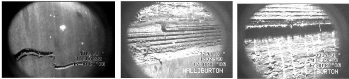
Fig. 10. Examples of failures detected by the video inspection. From left to right: Circumferential fracture of the pipe body, of the threaded coupling, and thread jump-out. From Osnes et al. (2007) .
