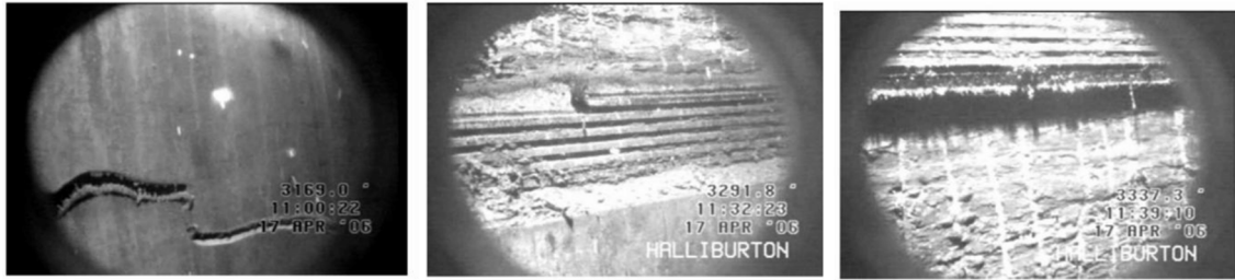
Fig. 10. Examples of failures detected by the video inspection. From left to right: Circumferential fracture of the pipe body, of the threaded coupling, and thread jump-out. From Osnes et al. (2007) .
