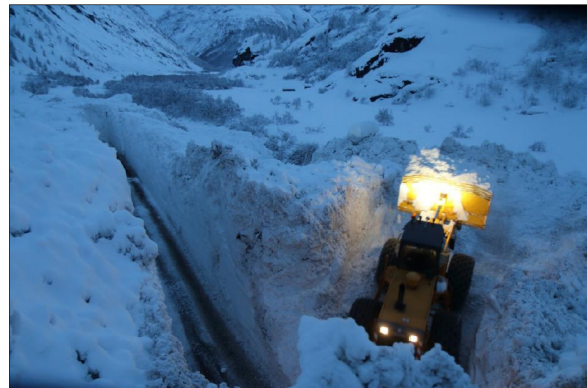
Figure 1: Removing snow on road RD 902 after exceptional snow avalanche occurred on 8th January 2018, Bérion, Savoie, France (courtesy of A. Duclos)
