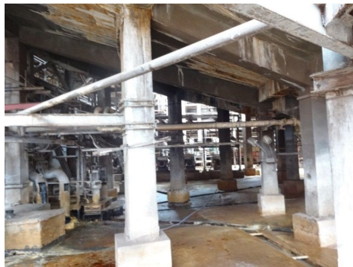
Figure 1. A RCC tertiary thickener structure of Alumina plant rests on concentric columns
