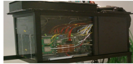
Fig. 20. Immersion cooling container prototype in Orange Labs
