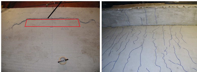
Figure 4: Thin slab failure mode: a) top face; b) bottom face
