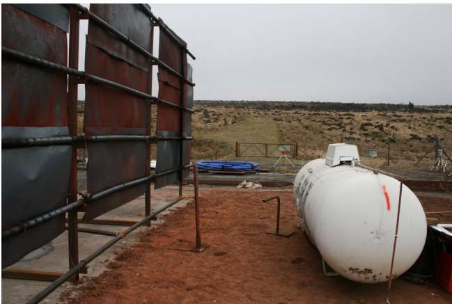
Fig. 1. Picture of tank located beside the wall fire simulator.
