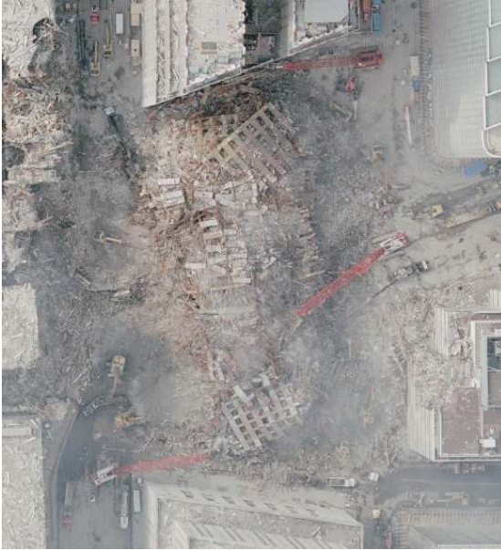
Figure 18: Aerial picture of WTC7 rubble pile during cleanup operation, cropped from [55]. Some almost undamaged facade walls parts are clearly visible, covering some much more shattered debris.
