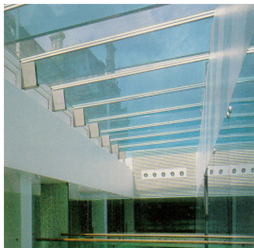
Fig 1: An example of structural glass : tempered beams supporting a glass roof in the Louvre museum
