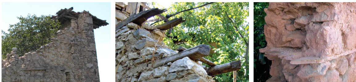
Figure 2: a) massive timber logs embedded in a partially collapsed masonry wall at Poggio Picenze (Italy); b) ladder-like timber bands inserted at regular spacing in Cumalikizik (Turkey) and c) planks insertion in a masonry wall in Kastamonu (Turkey) (Credit: Hofmann)
