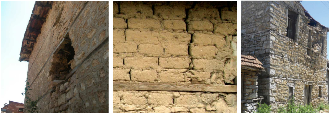
Figure 4: a) ladder-like insertions acting as lintels when partial collapse of a masonry wall occurred; b) preventing cracks propagation and c) restricting bending deflection (Credit: Hofmann)
