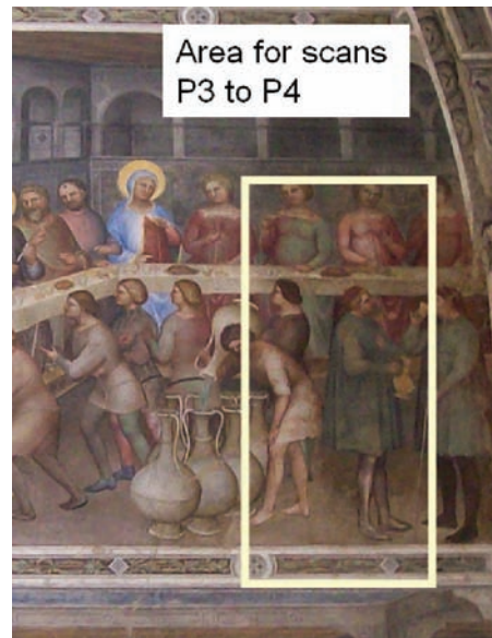
Portion of the north wall with delimitation of the scanned area. Real dimensions are approximately 1.5 m x 5 m.
