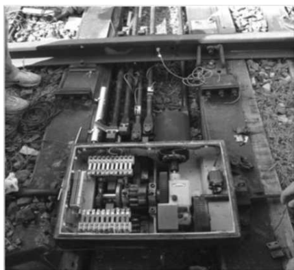
Figure 2. Electro-mechanical point machine.
