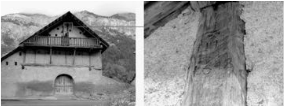
Fig. 2: Farmhouse, Val-des-Prés (05). Dating inscription details [IHS / 1648], on the western roof truss of the framework (photographs L. Shindo)
