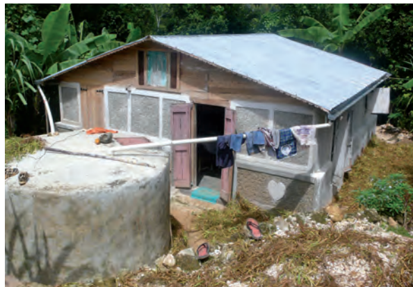
Below: some of the achievements of the project - houses and water tanks repaired in the framework of the project
