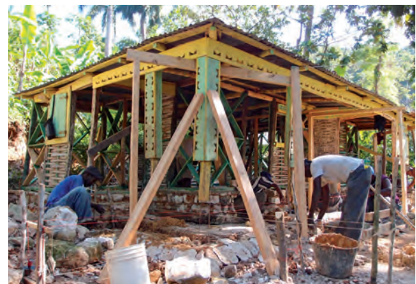
Above: Maison Joseph Dieujuste, Coupeau area, located a 6 hour walk from Carrefour City. Repair and improvement of the house. Propping of the structure, sawing of posts and construction of the stone foundation
