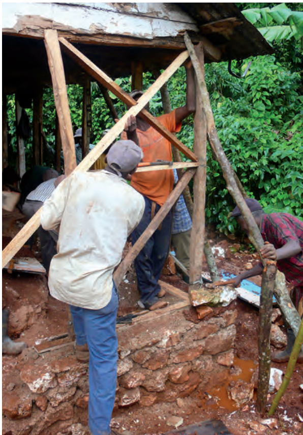
Below: training construction site in Cap Rouge, repair and reinforcement of existing structures
