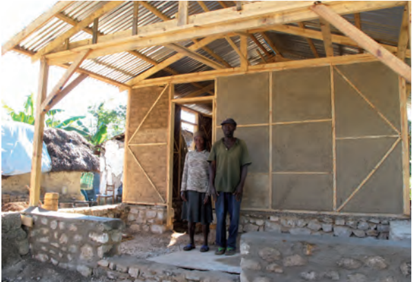
Below: Examples of wood-frame and brick houses, filled with moulded earth bricks
