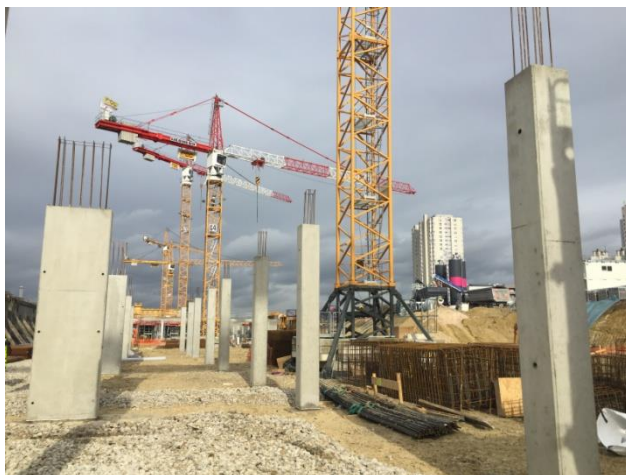
Figure I.9. Chapelle International Sogaris logistics hotel building site, 27 January 2016 Source: photo L. Dablanc
