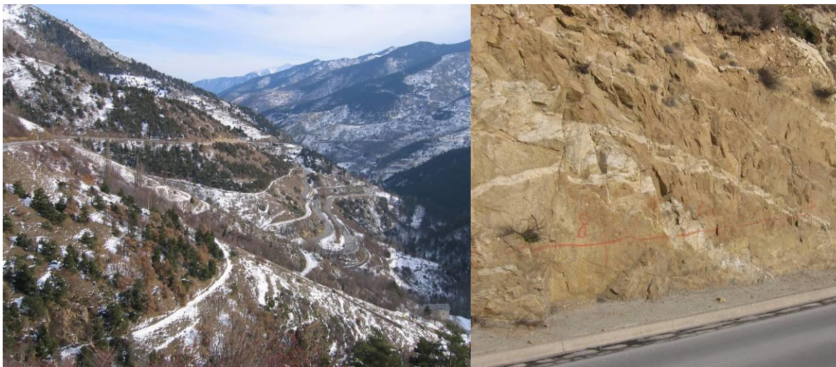
Fig. 1. Left: Panoramic view of the sector of Pallat, showing the existence of danger due to rock mass instability- Right: close-up of the fracture system at the road side outcrop, and measuring scanline.
