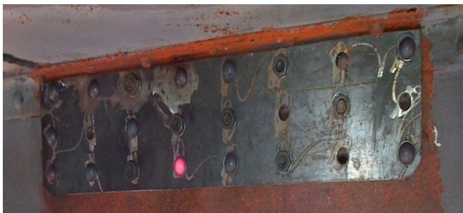
Figure 1. Additional riveted plate
