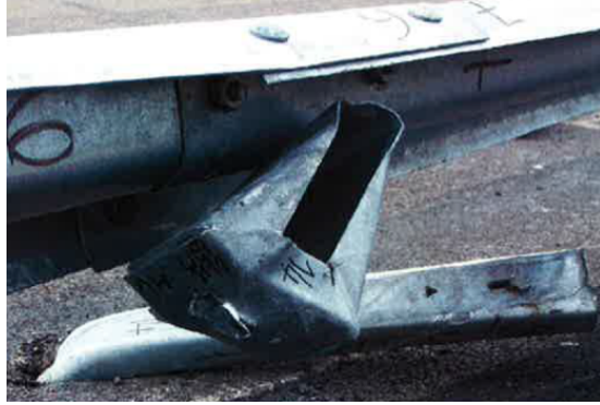
Figure 11: Bolts pull out failure of post-spacer connection
