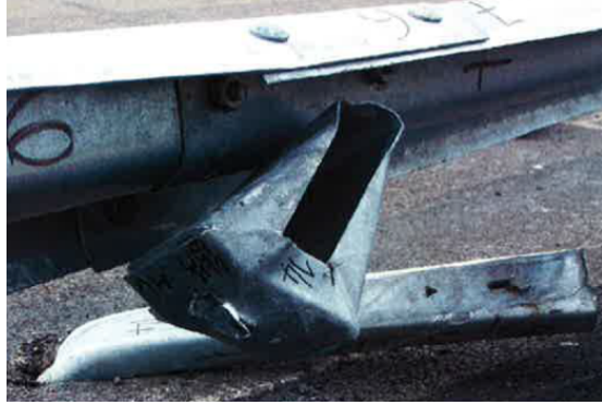
Figure 11: Bolts pull out failure of post-spacer connection
