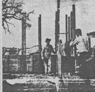
FORMS ARE HELD in alignment by vertical scaffolding tied by transverse rods. Holes left by removal of rods are plugged with dagga.
