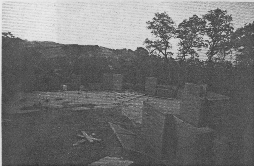
A Rammed Earth Works home isn't built in a day, but between sunrise and sunset, a lot of walls can go up. One worker handles the pneumatic tamper; one tills the pile of subsoil; another, on the tractor, carries dirt to the wall forms; a fourth sets up forms and takes them down.
