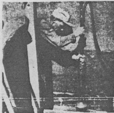
COMPRESSED AIR HAMMER with special head compacts soil. Each horizontal run, about 4 in. deep after tamping, is rammed in one continuous operation for each wall.
