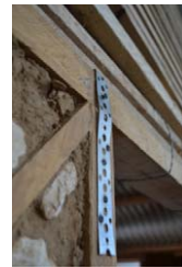
(e) HTI 300%: Connection–Location 7: South transv. wall
