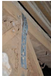
(g) GUA 390%: Connection– Location 7: South transv.wall
