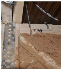
(j) GUA 390%: Ligature wire–Location 8: West shear wall
