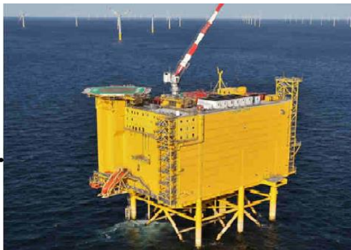
Assemble all the currents from all wind turbines in DC form and deliver it over the sea
