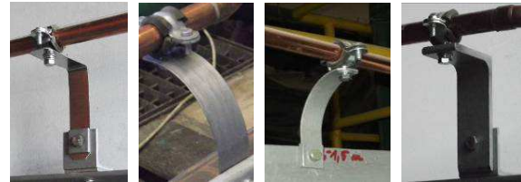
Figure 4. Flat springs (from the left) FS2, FS3, FS4, and FSR for supporting the pipeline
