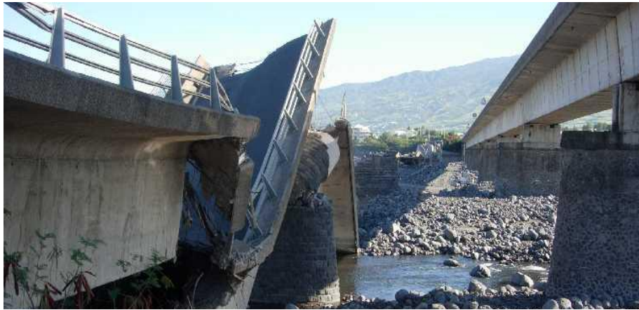
Fig. 1 Collapse induced by scour of the RN1 bridge on the St Etienne River, Reunion Island (Feb 2007)
