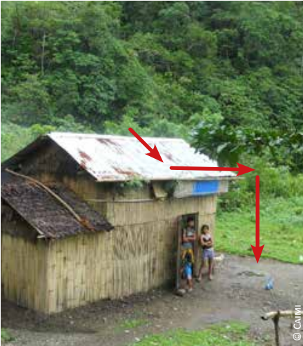
Philippines: rainwater is redirected away from the building thanks to a bamboo gutter
