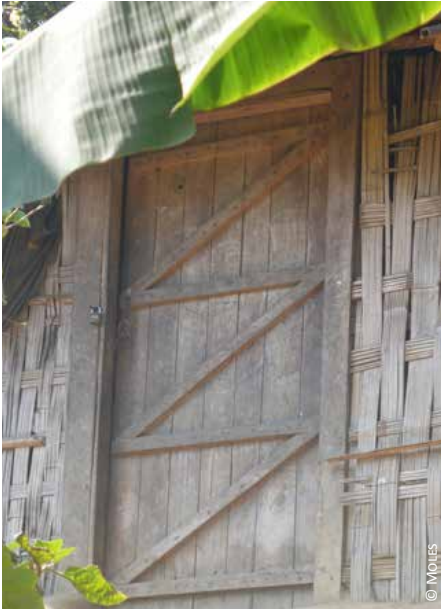
Bangladesh: bracing on timber door shutter
