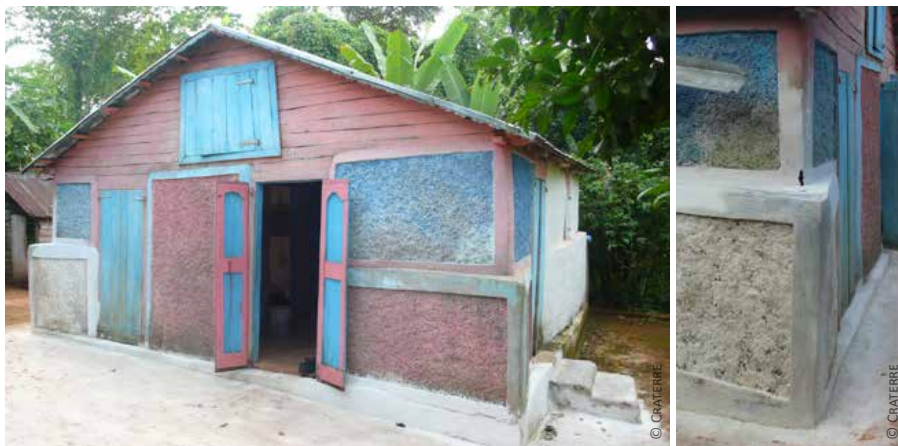
Haiti, sharp corner reinforcement: 1) view on the building and 2) zoom on the corner
