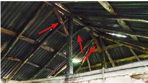
Haiti: diagonal bracing connecting the king post to the ridge beam
