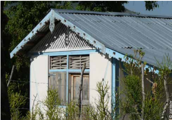
Haiti: 3) perforated panels above the windows and on the upper part of the gable end wall of a house rebuilt after 2010 earthquake
