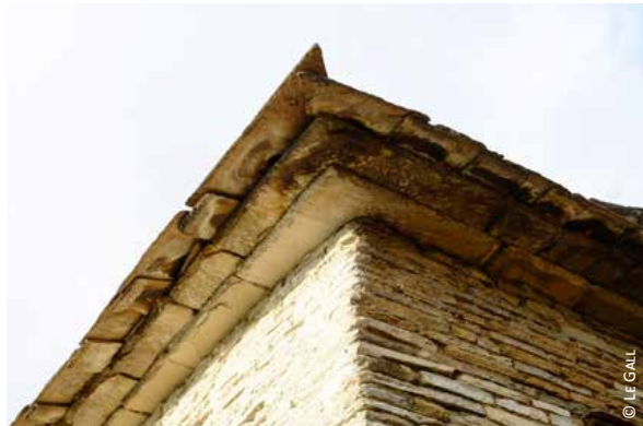
Nepal, after the 2015 M 7.8 Gorkha earthquake: 1) flat stone coping
