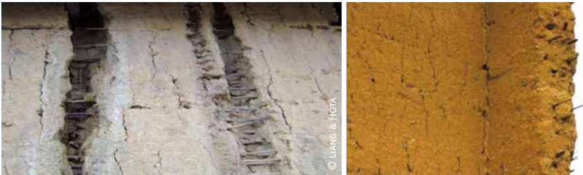
China: 3 & 4) thin bamboos embedded into the mass of the rammed earth walls of XI century tulou houses in Fujian province
