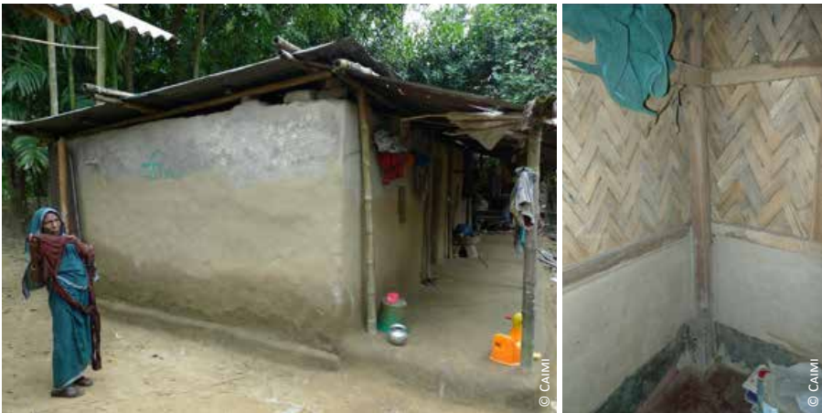
Bangladesh: 2) after flooding, people keep on living inside the house even if the back walls have been damaged; 3) half earthen wall with indoor independent structure for the roof
