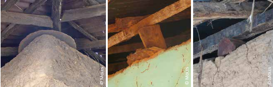
Guinea Bissau, anti-termite barrier: 1) curved metal piece; 2) recycled iron sheet; 3) hard wood
