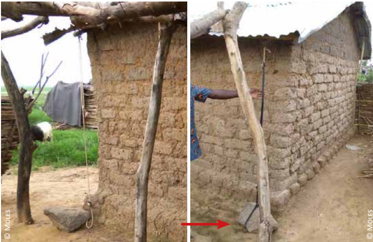
Benin: 4) a rope tied to the roof structure provides a potential anchoring system 5) during the windy season, ropes are anchored to big stones at the corners of the building
