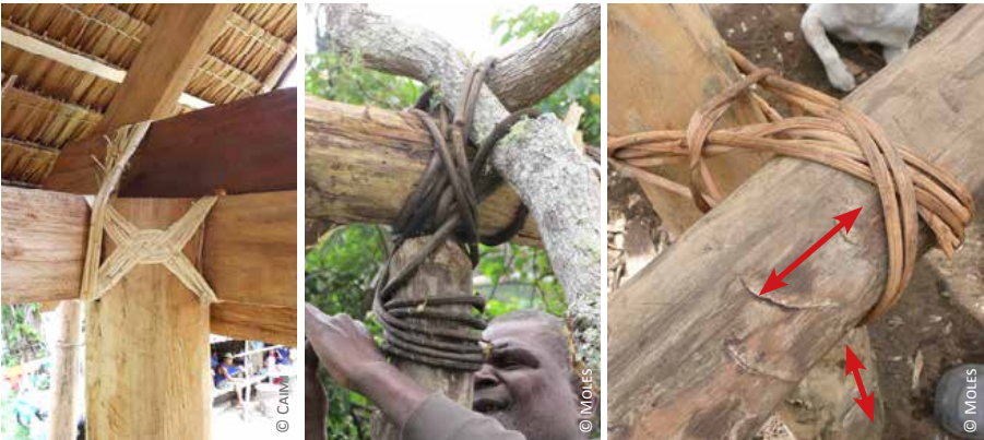
1) Philippines: rattan ties for connecting posts, ring beam and roof structure Vanuatu: 2) ties with creepers; 3) movements of the structural elements under wind loads
