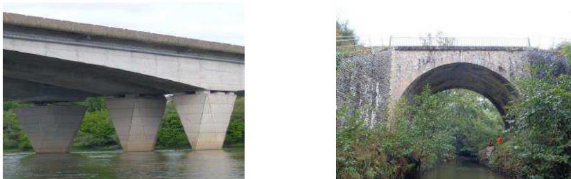
Fig. 2. (Left) Investigated site on the A71 motorway double viaduct next to Orléans (France) over Loire river (one support with its 3 piers). (Right) Railway bridge, investigated site over the Aurence River close to Limoges (France).
