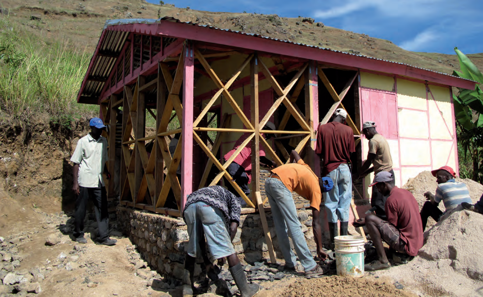
Above: training construction worksite, Belle Fleur: wood frame house filled with Ti-woch and earth bricks
