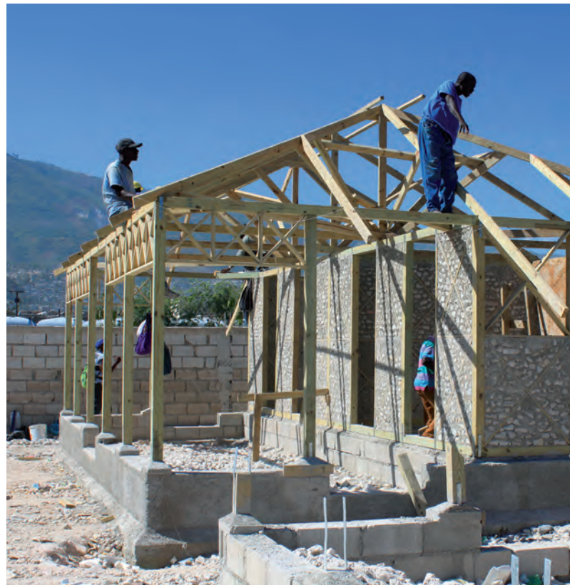
Wood frame wall panels filled with masonry debris
