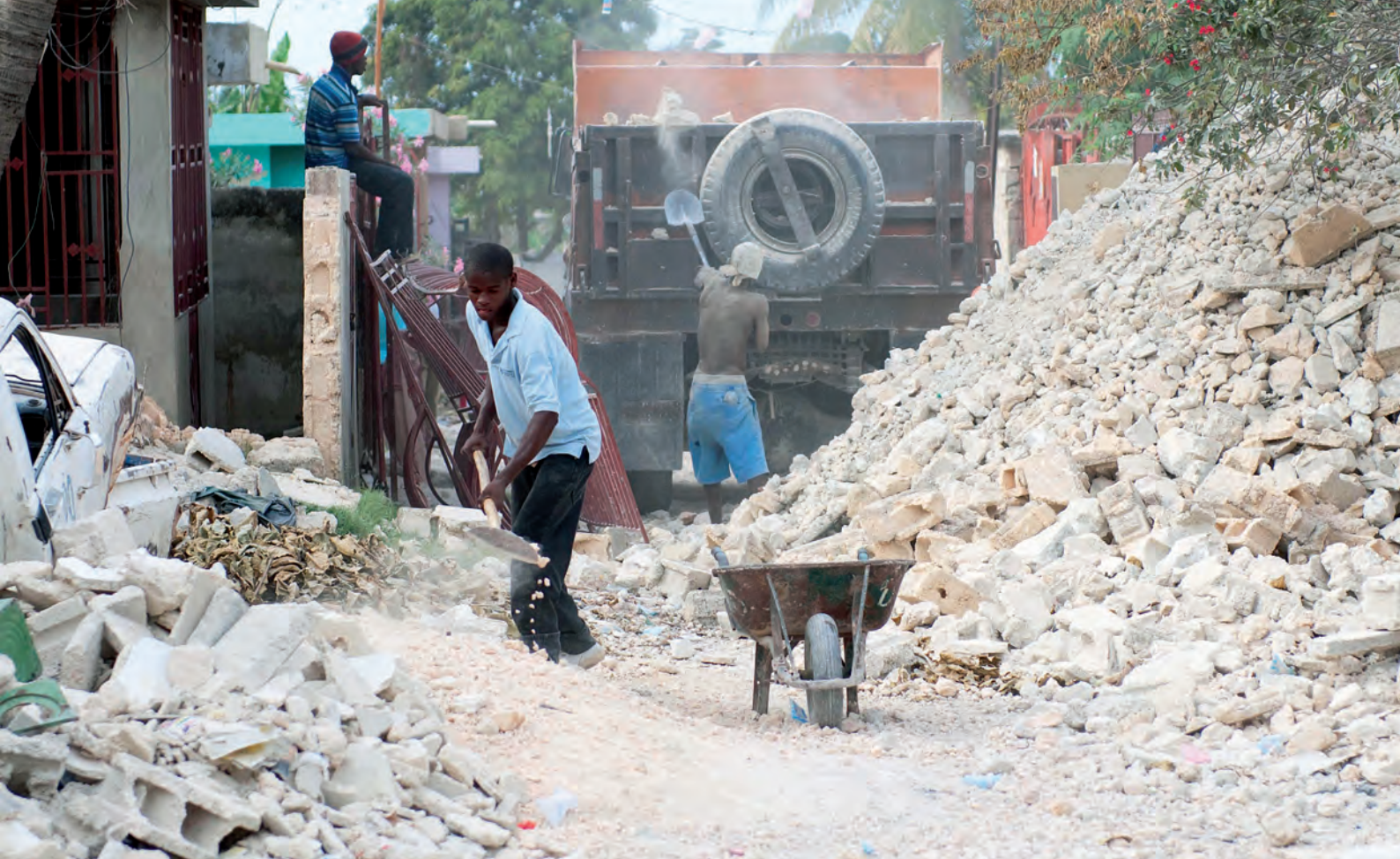
Above: clearing and collection of earthquake debris in the streets of Port-au-Prince
